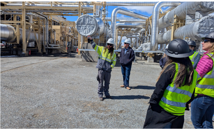
A Fervo Energy engineer explains the operation of Cape Station's geothermal power plant, highlighting heat-exchange systems and power-generation infrastructure. Photo by Brian Gootee
