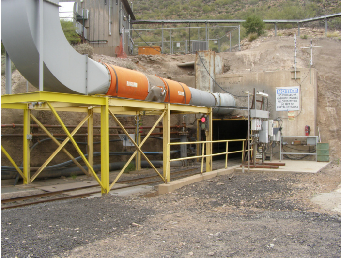
Figure 10. Entrance to Never Sweat Tunnel with ventilation system (June 2015).
